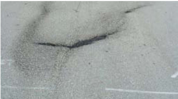
Figure 1 Slippage Failure Due to Poor Bond Between Layers
