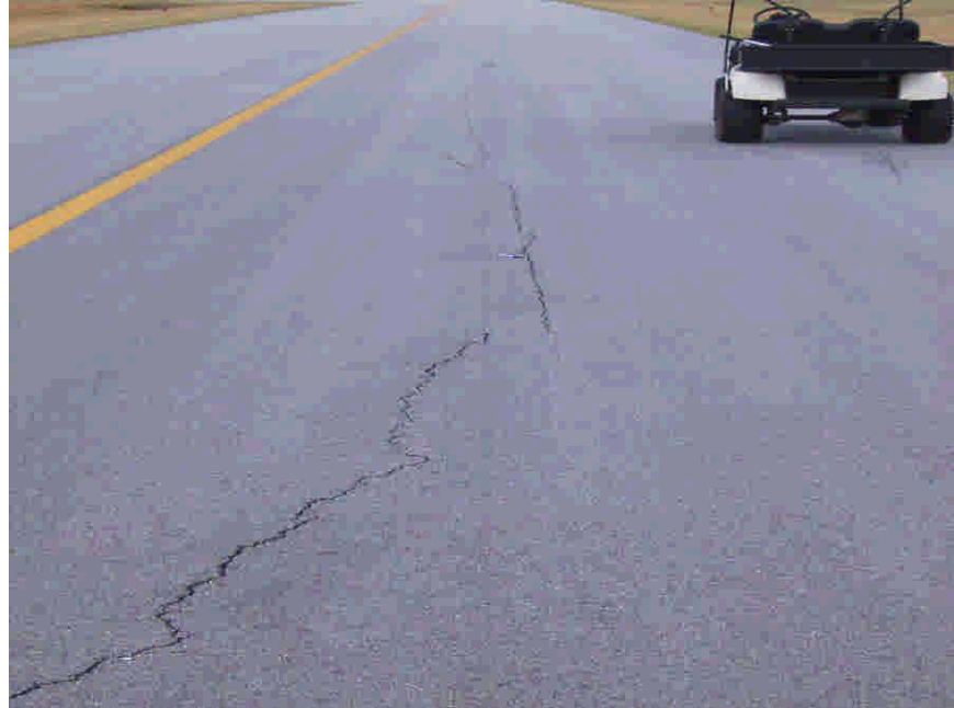
Figure 14: Longitudinal Cracking Along Taxiway, 9.5mm A
