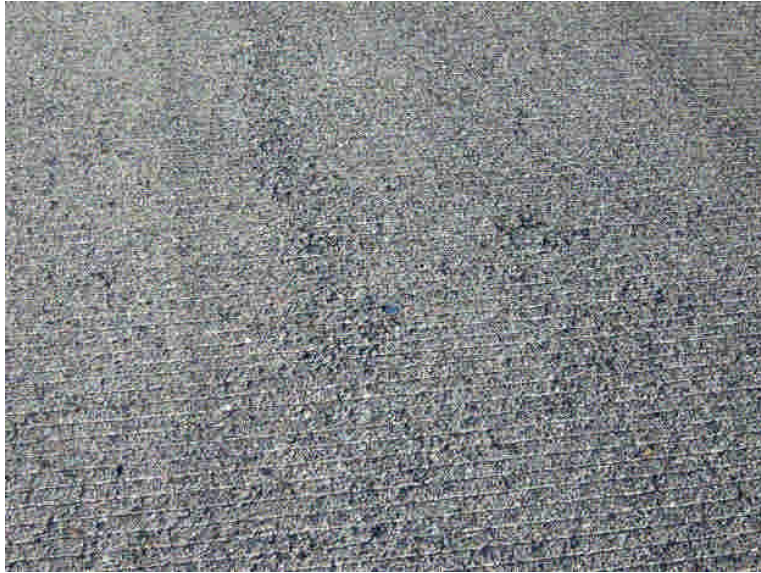
Figure 28: Ravelling of Pavement
