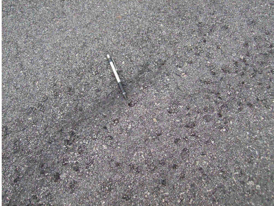
Figure 16: Pavement Distress Caused by Vapor Pressure, 9.5mm A
