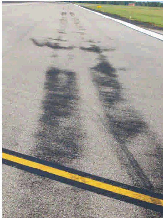
Figure 29: Bleeding and Blistering in Runway
