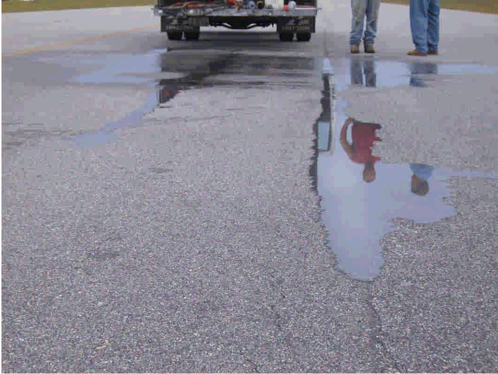
Figure 21: Water Ponding along Longitudinal Joint (Right) and Wheel Rut (Left)
