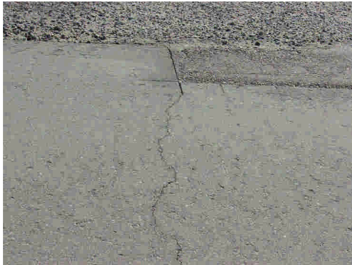
Figure 9: Transverse Crack Initiated at Construction Joint
