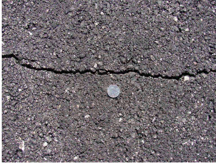
Figure 12: Transverse Crack and Surface Texture on Runway 07/25
