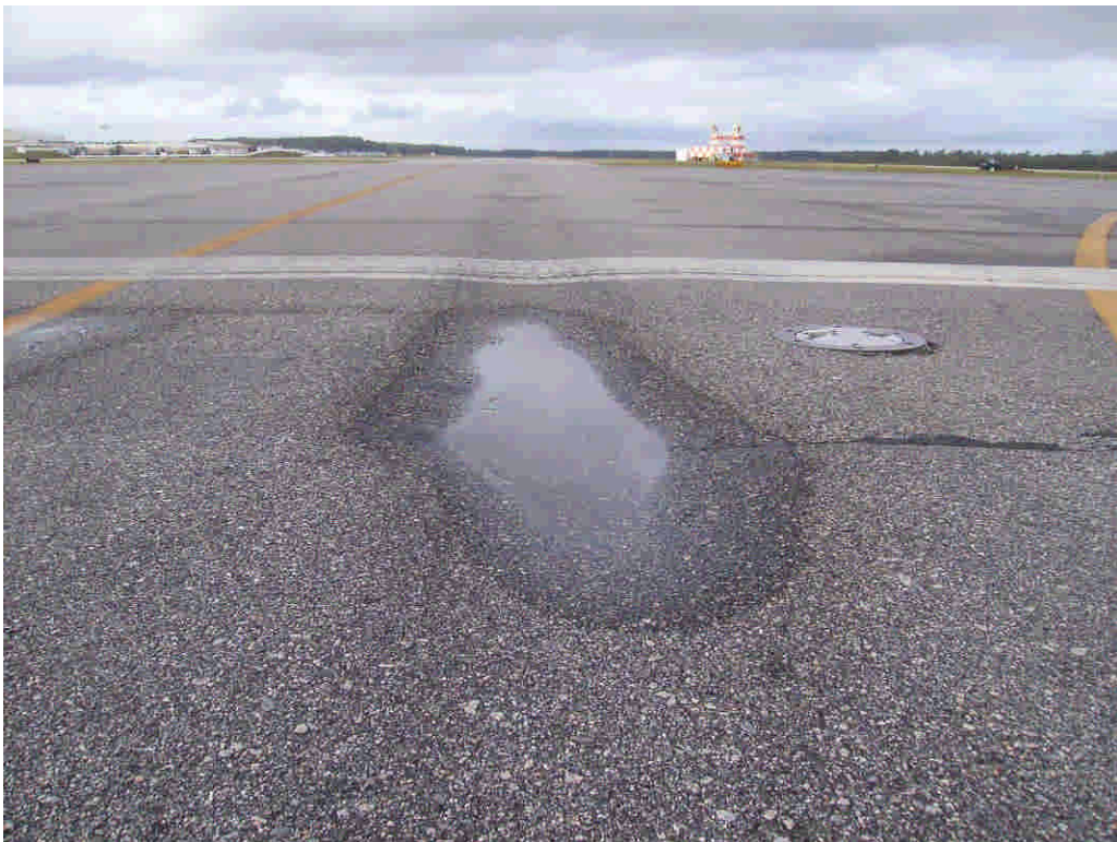
Figure 22: Rutting on Taxiway Alpha
