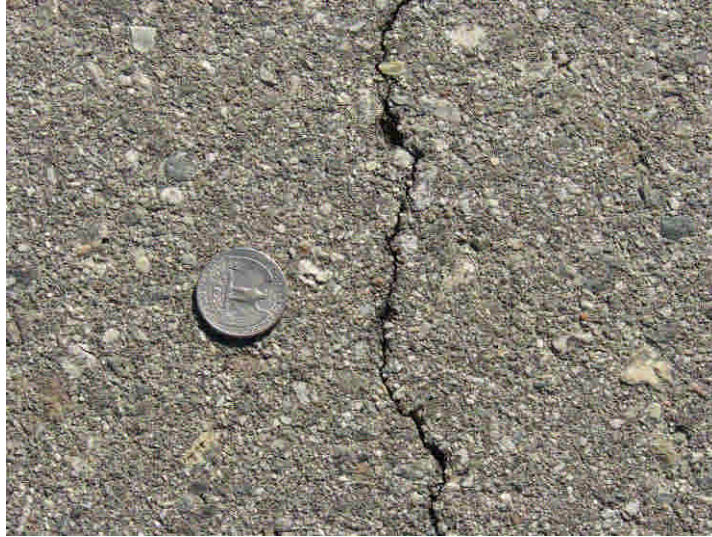
Figure 10: Close-up of Transverse Crack and Surface Texture
