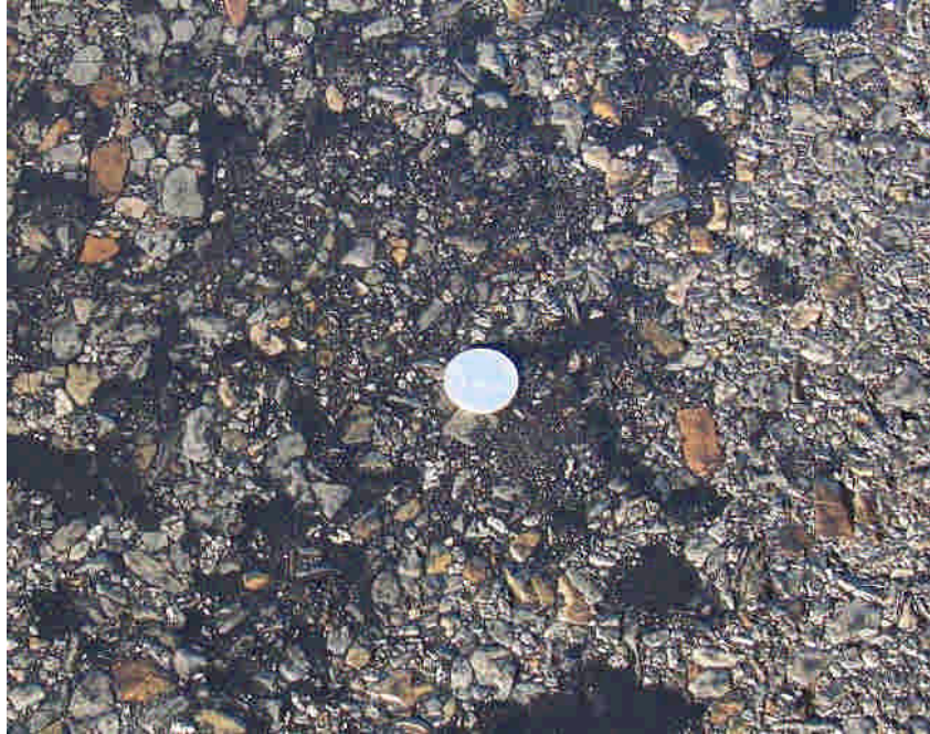
Figure 17: Bleeding on Assault Strip
