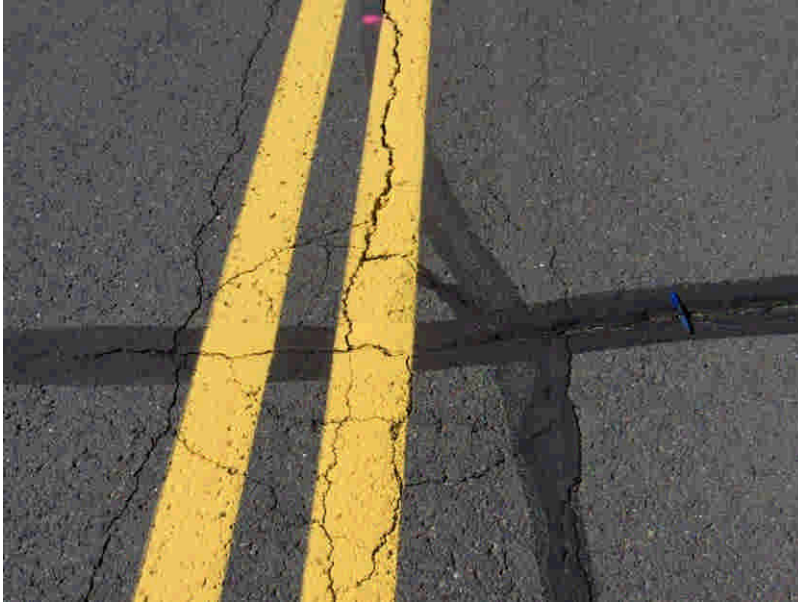
Figure 35: Intersection of Longitudinal Crack and Transverse Crack
