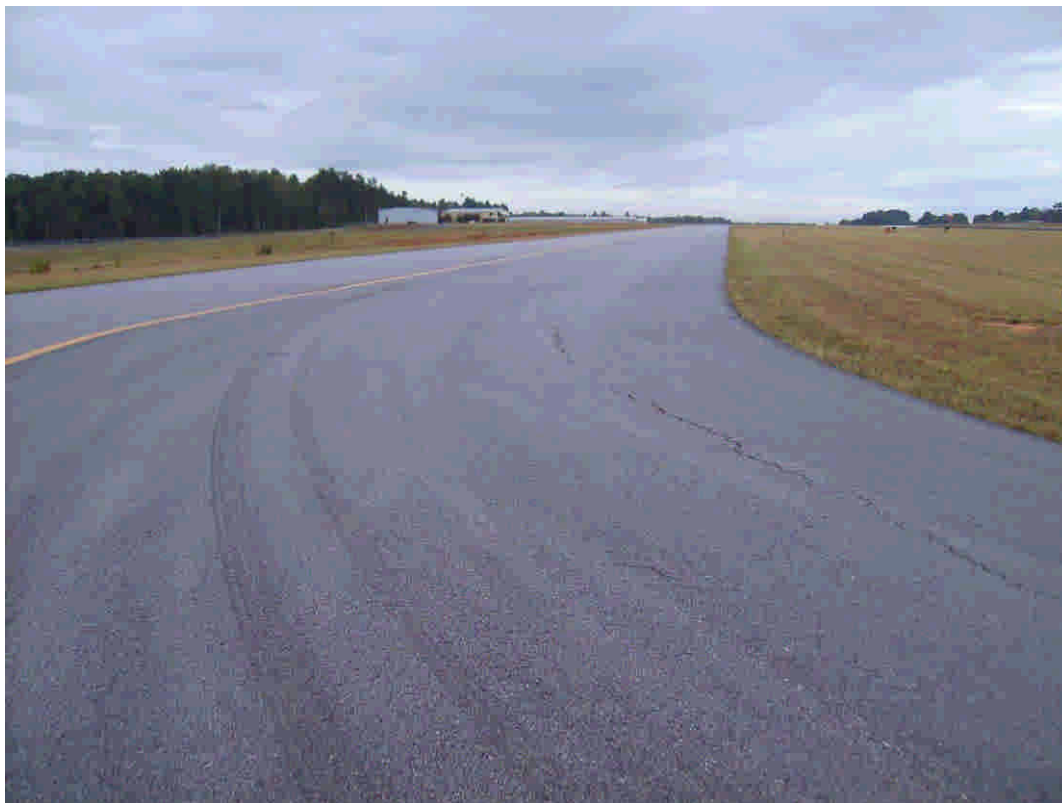
Figure 15: Cracking in the Turnout to Taxiway, 9.5mm A.
