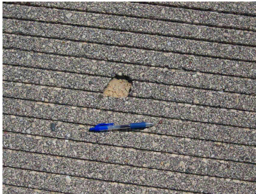
Figure 27: Example of Occasional Popout and Performance of Grooves
