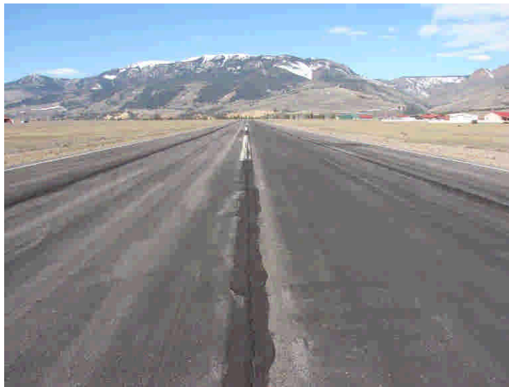
Figure 11: Runway 07/25 Showing Longitudinal Joint Cracks
