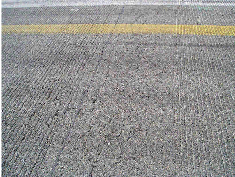
Figure 32: Transverse Cracking in Ungrooved Section of Runway 11/29
