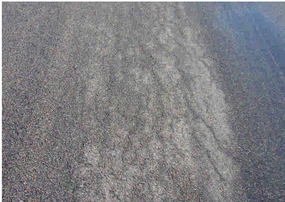
Figure 20: Cracking Near End of Runway
