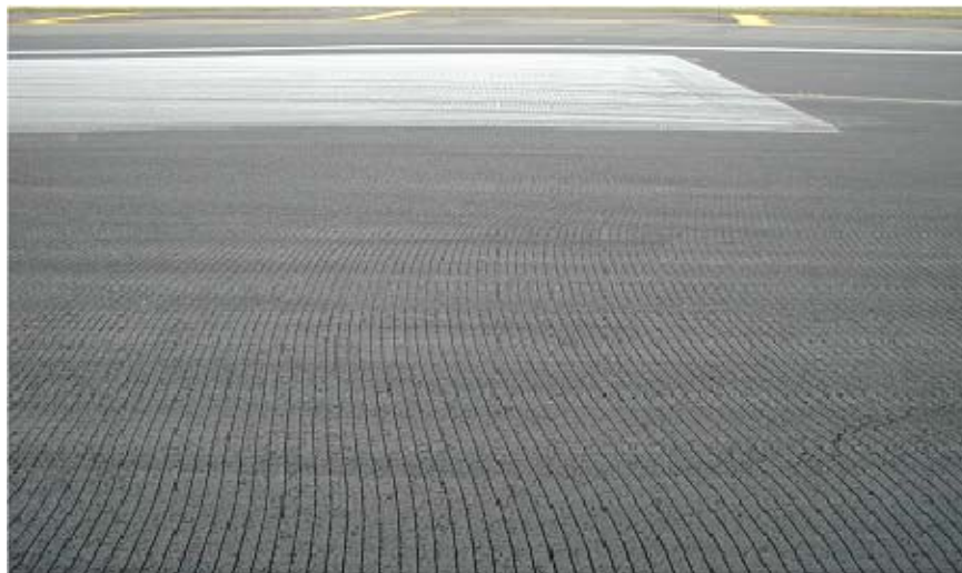
Figure 1.2 – Slippage at High-Speed Taxiway (“Curved” Grooves Indicate Slippage, Bognacki et al., 2007)
