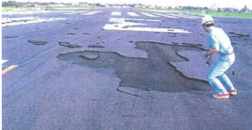
Figure 1.1 – Slippage Failure due to Loss of Bond at Nagoya Airport (from Tsubokawa et al., 2007)
