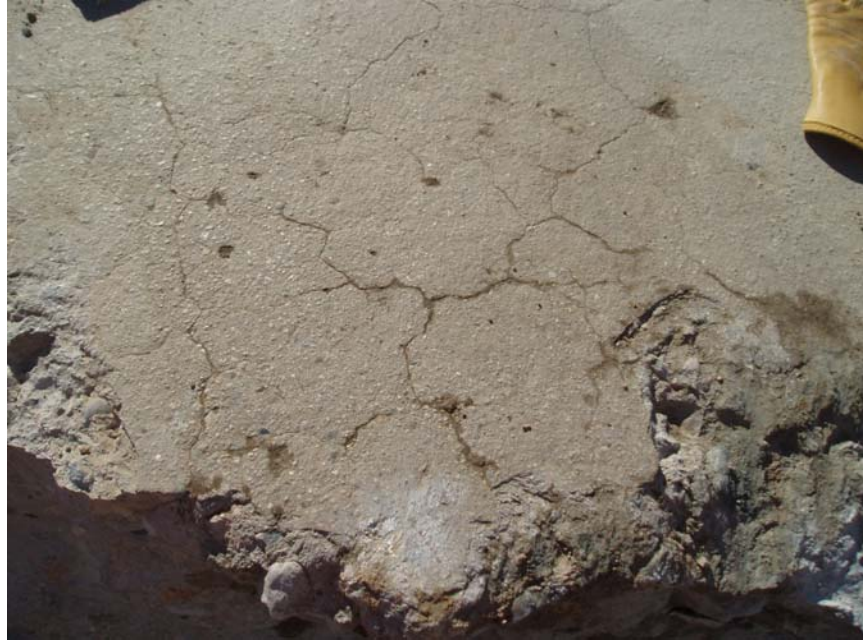
Figure 2. Map-Cracking of Pavement Surface for Edwards AFB
