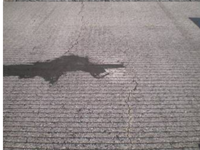
Figure B-34. Cracking, raveling and patching on Runway 30 near Taxiway Foxtrot, Colorado Springs Airport.
