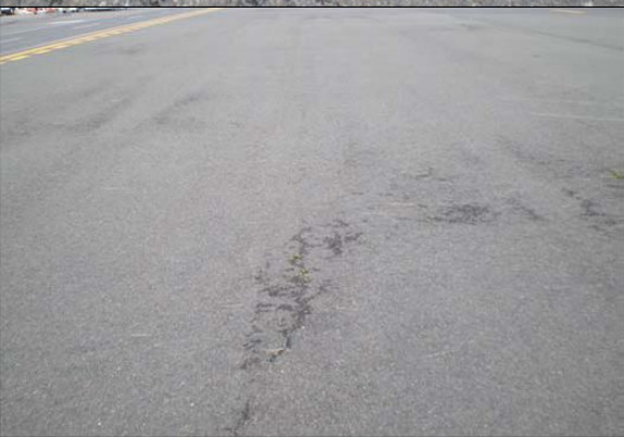
Figure B-12. FedEx Cargo area apron and south outer Taxiway K, Boston Logan Airport. Milled and overlaid with P-401 asphalt concrete in 2000. Asphalt concrete shows low severity cracking and raveling.
