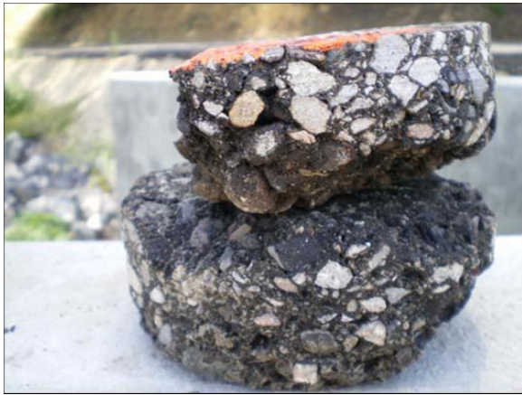
Figure B-45. Core #2 from Friedman Memorial Airport. Note deterioration of the asphalt concrete between the surface and binder course lifts. Note the stripping of the asphalt cement from the aggregate at the surface of the binder course lift.
