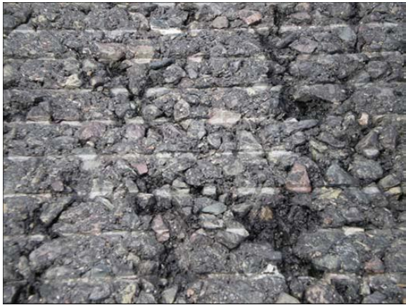
Figure B-21. Boston Logan Runway 06/27 near Taxiway C. Close-up of location shown in Photograph B-20. Note the missing fine aggregate particles and stripping of the asphalt cement from the coarse aggregates.
