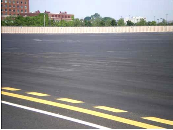
Figure B-19. Taxiway J and asphalt overrun at the end of Runway 14, Boston Logan Airport. Asphalt concrete pavement constructed in 2006. No evidence of any raveling or stripping.
