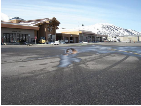
Figure B-41. Apron pavement looking west towards the terminal building, Friedman Memorial Airport. Rutting due to aircraft gear loading in front of the terminal building.
