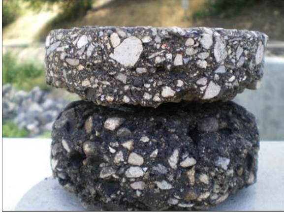
Figure B-44. Core #1 from Friedman Memorial Airport. Note deterioration of the asphalt concrete between the surface and binder course lifts.
