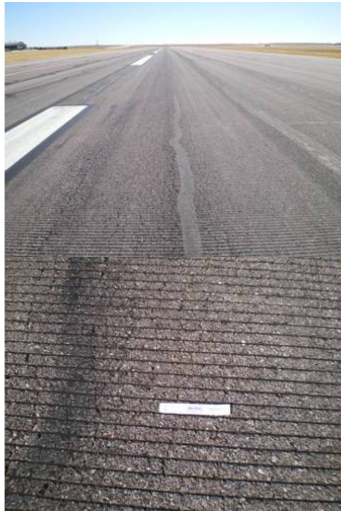
Figure B-36. Runway 12/30 looking south at Taxiway MIL, Colorado Springs Airport. Note the over-band crack sealing approximately 10 feet west of the runway centerline in the primary wheel path area. Low severity fatigue type cracking on either side of the sealed crack.
