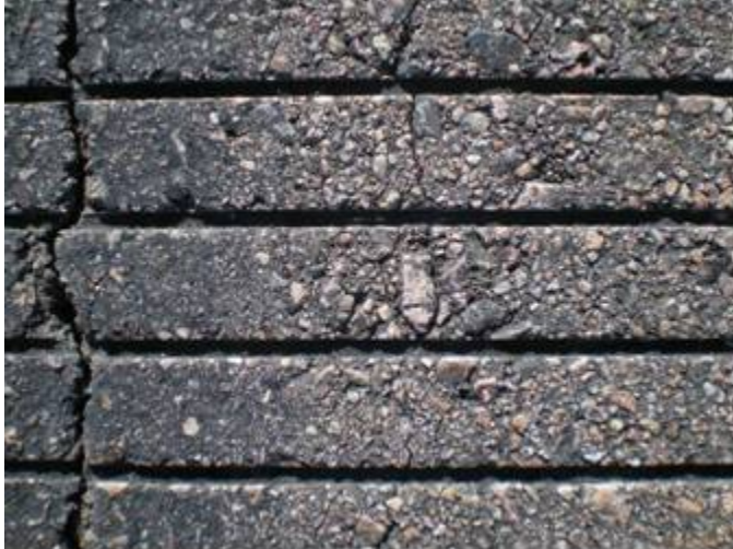
Figure B-29. Close-up of slight segregation and secondary cracking near the low severity longitudinal construction joint crack on Runway 17L/35R, Colorado Springs Airport.
