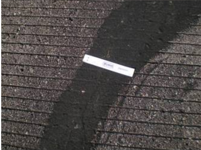
Figure B-31. Large over-band of crack on Colorado Springs Runway 12/30.
