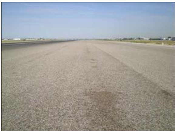
Figure B-2. Boise Runway 10L/28R looking east. The stained area is offset from the paving joint in the permeable friction course. Airport staff indicate that the staining may be pumping from a joint in the underlying base asphalt concrete.
