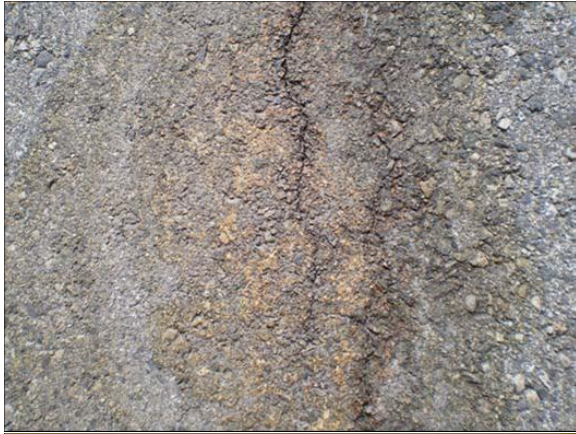
Figure B-7. Runout area north of Boise Runway 28R near the south edge of the pavement. Severe staining, cracking and some raveling of the asphalt concrete. The surface in this area is P-401 asphalt concrete.
