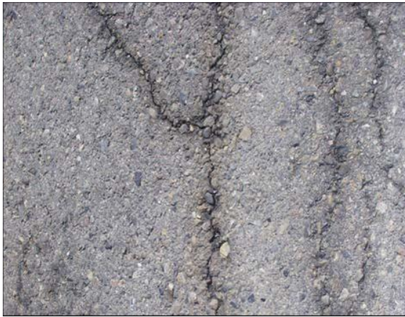
Figure B-42. Close-up of cracking and raveling of the pavement surface.
