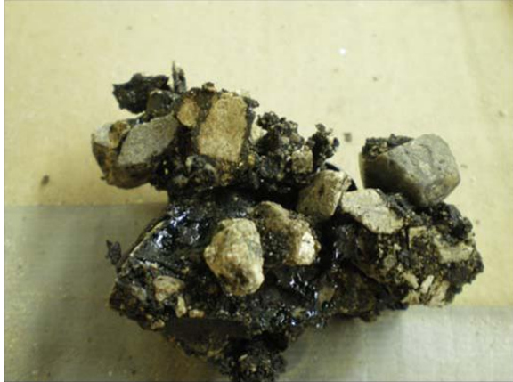
Figure B-8. Close-up of an asphalt sample taken from a core of the runway at Boise Airport. Note the complete stripping of the asphalt cement from the aggregate.
