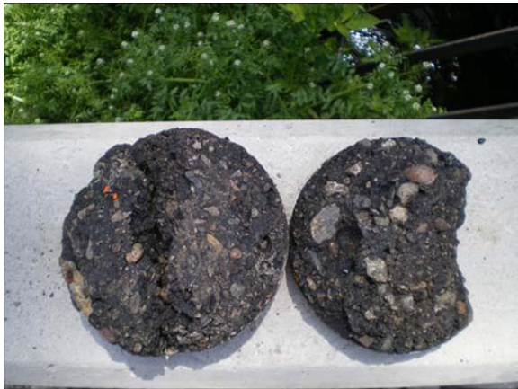
Figure B-48. Core #4 from Friedman Memorial Airport. Close-up of the bottom of the surface course life (left side of photograph) and top of the binder course life (right side of the photograph). Note the stripping of the asphalt cement from the coarse aggregate.
