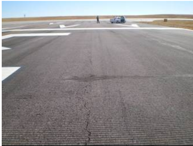
Figure B-32. Mid-mat longitudinal cracking and moderate severity transverse crack near the south end of Runway 30, Colorado Springs Airport.
