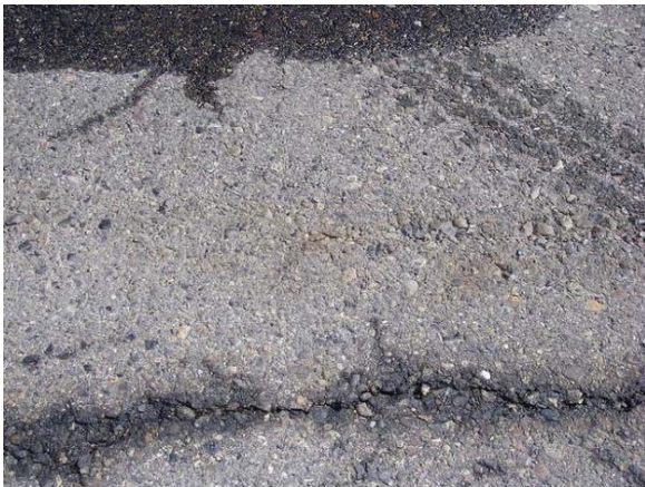
Figure B-43. Close-up of cracking and raveling of the asphalt concrete at the cracks.
