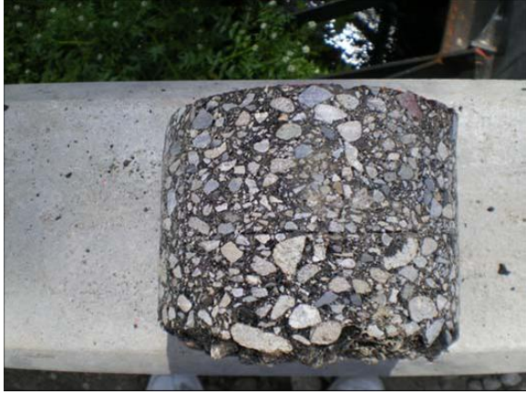
Figure B-50. Core #6 from Friedman Memorial Airport. Surface and binder course intact. Some open structure is evident at the bottom of the core but may be due to poor compaction of the lower lift.
