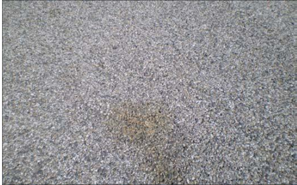
Figure B-3. Close-up of the staining on the surface of the pavement at Boise, Idaho Airport.
