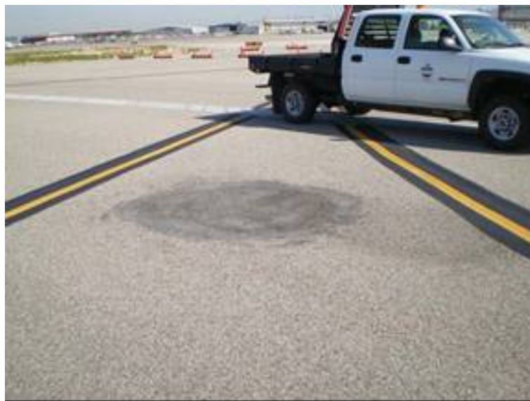
Figure 8. Boise Runway 10L/28R looking toward the intersection of Taxiway E. This shows a patched area and an initial depression and shoving noticed in 2006. Aircraft landing on Runway 10 used this taxiway for relatively high speed exits to the terminal area. This resulted in some fairly high braking forces. No additional distress has been observed.
