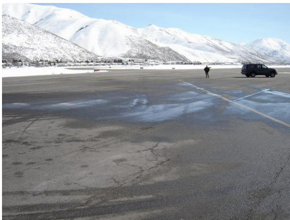
Figure B-40. Apron pavement looking east, Friedman Memorial Airport. Rutting and depressions in the apron pavement in front of the terminal building.
