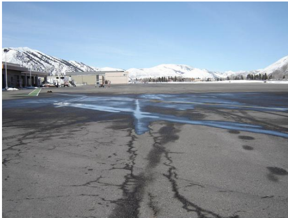
Figure B-39. Apron pavement looking north, Friedman Memorial Airport. Alligator cracking and rutting (transverse to the photograph) on the apron in front of the terminal building.
