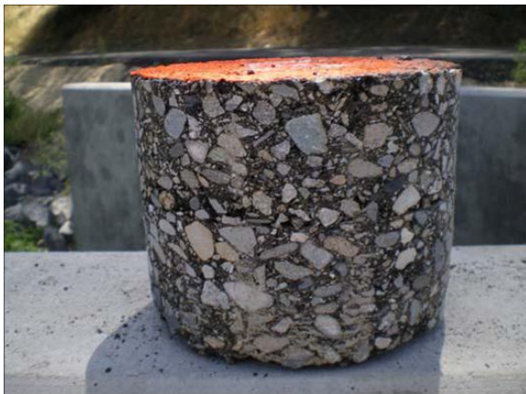
Figure B-49. Core #5 from Friedman Memorial Airport. Intact surface and binder course. Some deterioration between the lifts is evident on the left side of the photograph.
