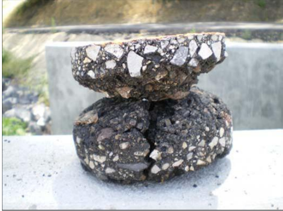
Figure B-47. Core #4 from Friedman Memorial Airport. Surface and binder course has lost some of the aggregate.
