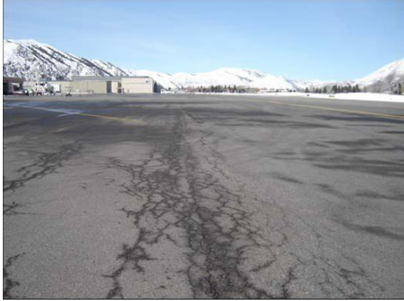
Figure B-38. Apron pavement looking north, Friedman Memorial Airport. Alligator cracking at a longitudinal construction joint.
