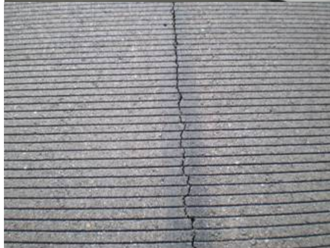
Figure B-28. Close-up of low severity longitudinal construction joint crack on Colorado Springs Runway 17L/35R.
