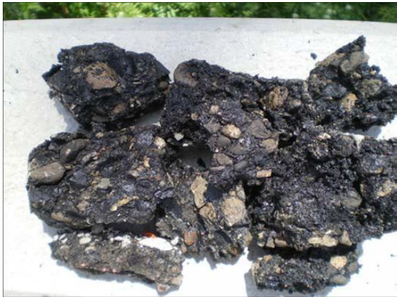
Figure B-46. Core #3 from Friedman Memorial Airport. The core was not able to be extracted in a solid piece. Note the stripping of the asphalt cement from the aggregate.
