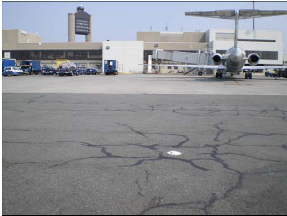
Figure B-14. Apron area in front of Boston Logan B Concourse near Gate B-28. Random pavement surface cracking. Photograph taken in a low area of the pavement. Deicing fluid from the gate deicing operation flows onto the asphalt concrete at this location. White dot indicates core location.
