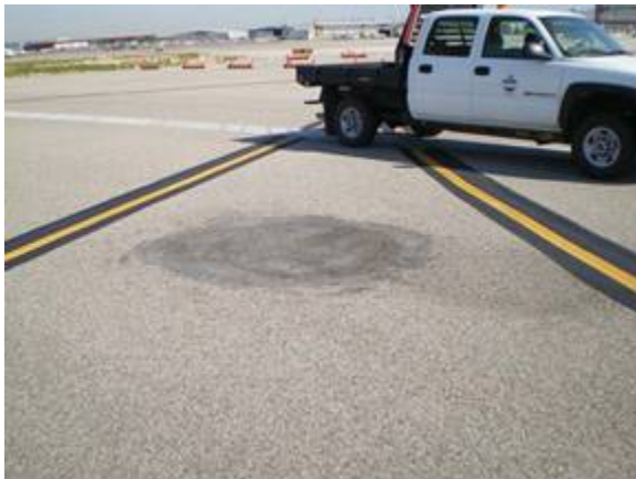
Figure B-1. Boise Runway 10L/28R looking toward the intersection of Taxiway E. This shows a patched area and an initial depression and shoving noticed in 2006. Aircraft landing on Runway 10 used this taxiway for relatively high speed exits to the terminal area. This resulted in some fairly high braking forces. No additional distress has been observed.
