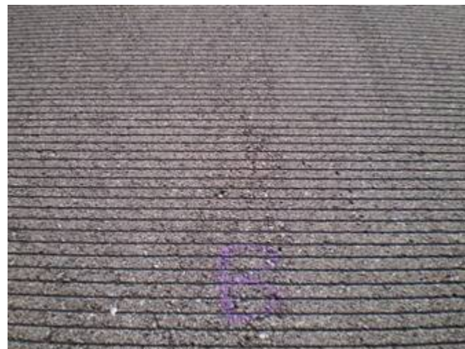
Figure B-33. Close-up of raveling and cracking about 10 feet west of the Runway 30 centerline, Colorado Springs Airport. Location selected for coring.
