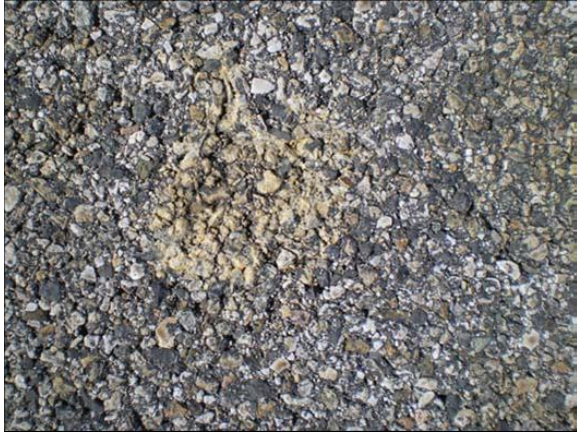
Figure B-4. Close-up of the staining on the surface of the pavement at Boise, Idaho Airport.
