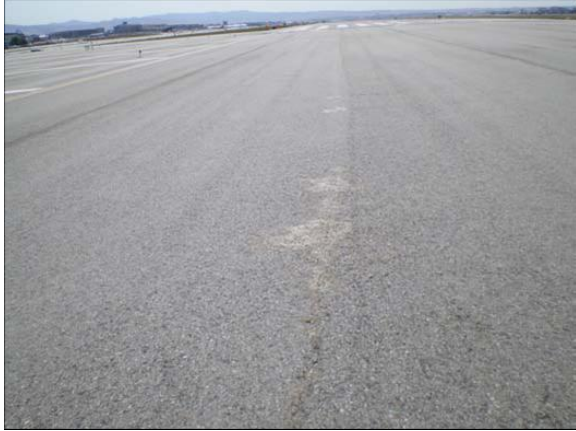
Figure B-6. Boise Runway 10L/28R north of Taxiway M. Note the staining along the longitudinal joint and low severity cracking in the foreground.
