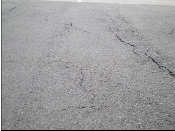
Figure B-16. Inner Taxiway area in front of Boston Logan B Concourse near Air Canada Gate 3. This area was milled and overlaid with 3 inches of P-401 asphalt concrete in 2000. Note the significant cracking, raveling and exposed aggregate.
