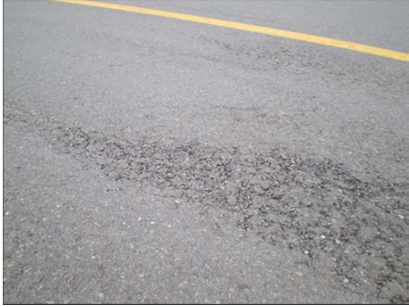
Figure B-22. Boston Logan Taxiway K near Taxiway L. Mill and overlay of 2.5 inches of P-401 asphalt concrete in 2001. This asphalt concrete includes the Bitumar AC-20 and liquid antistripping additive. Note the raveling and stripping of the asphalt cement from the coarse aggregate.
