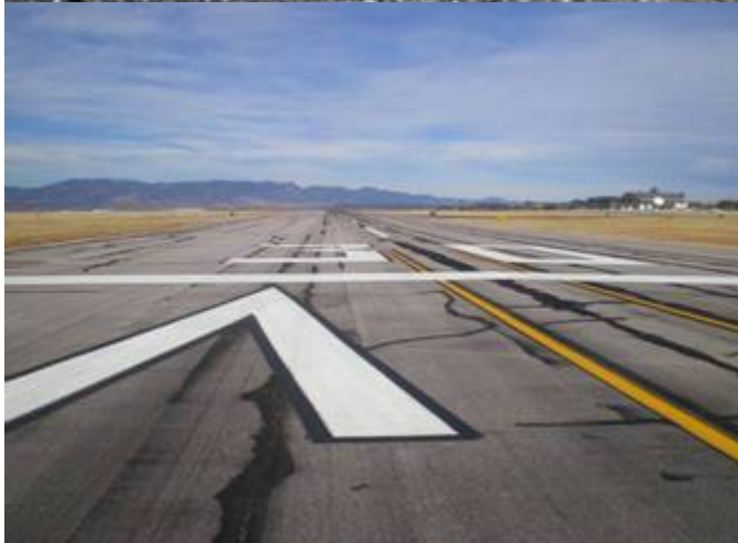
Figure B-30. Colorado Springs Runway 12/30 Looking north from the Runway 30 End. Most cracks including the primary longitudinal construction joint cracking has been sealed with hot-poured rubberized asphalt using an over-banding technique.
