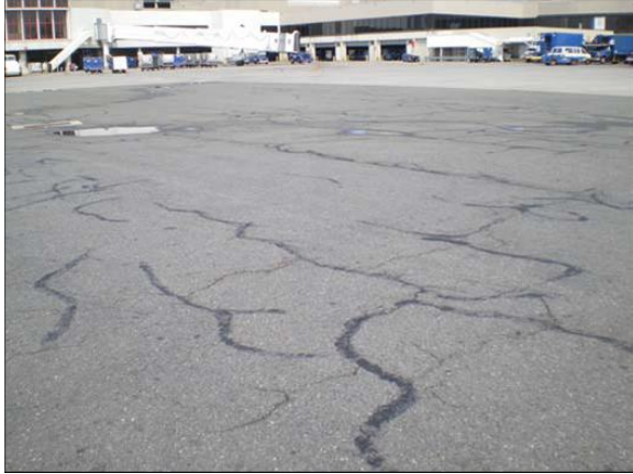
Figure B-13. Apron area in front of Boston Logan B Concourse near Gate B-28. This pavement was rehabilitated in 1981 consisting of a mill and overlay of 4 inches of P-401 asphalt concrete. Some of the cracking has been sealed but there are also many unsealed cracks. Aircraft anti-icing chemicals run onto this area of asphalt from the adjacent concrete apron pavement.
