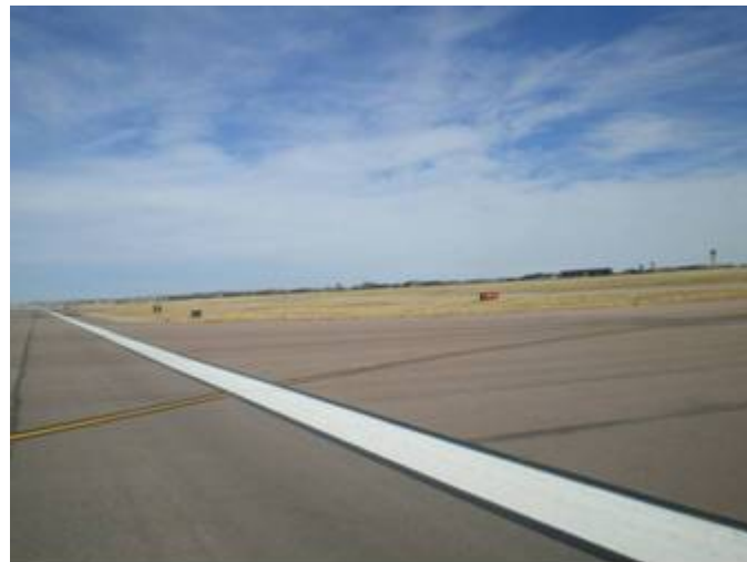
Figure B-27. Colorado Springs Runway 17L/35R looking east at intersection with Taxiway Hotel. The pavement is new and the only distresses present at this location are low severity longitudinal construction joint cracks.
