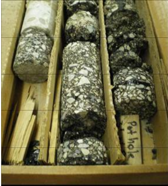
Figure B-9. Typical core taken from Boise Runway 10L/28R. The permeable surface course is on the right side of the photograph and is intact. Directly below the surface the asphalt concrete is stripped and deteriorated. The asphalt in the center of the box is the old surface below the asphalt concrete placed in 2000.
