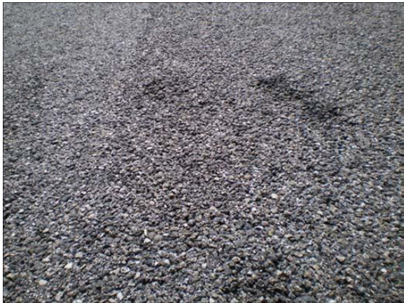
Figure B-5. Boise Runway 10L/28R near Taxiway B. Area to the right has older permeable surface course showing some signs of raveling. Pavement in the left of the photograph was paved in 2000.
