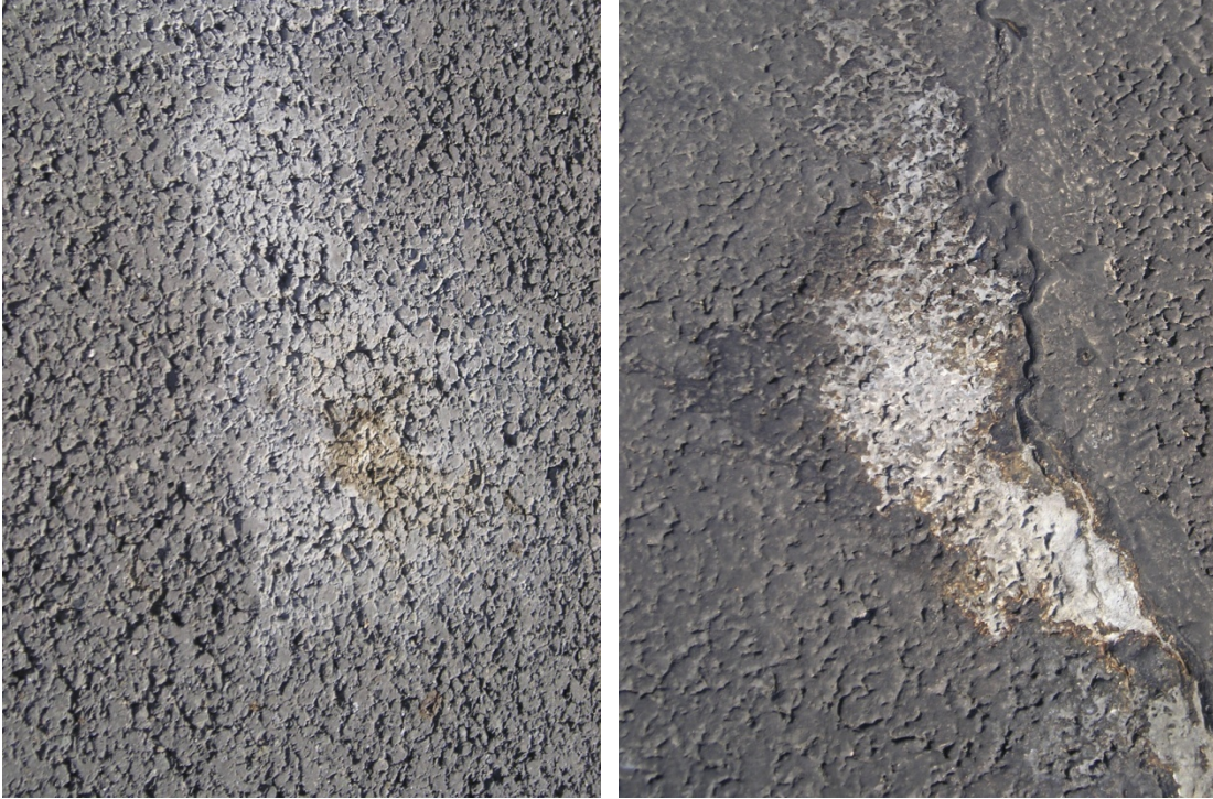
FIGURE 3.8 Surface Staining from Moisture Damage in Underlying Layers at Harbin.
