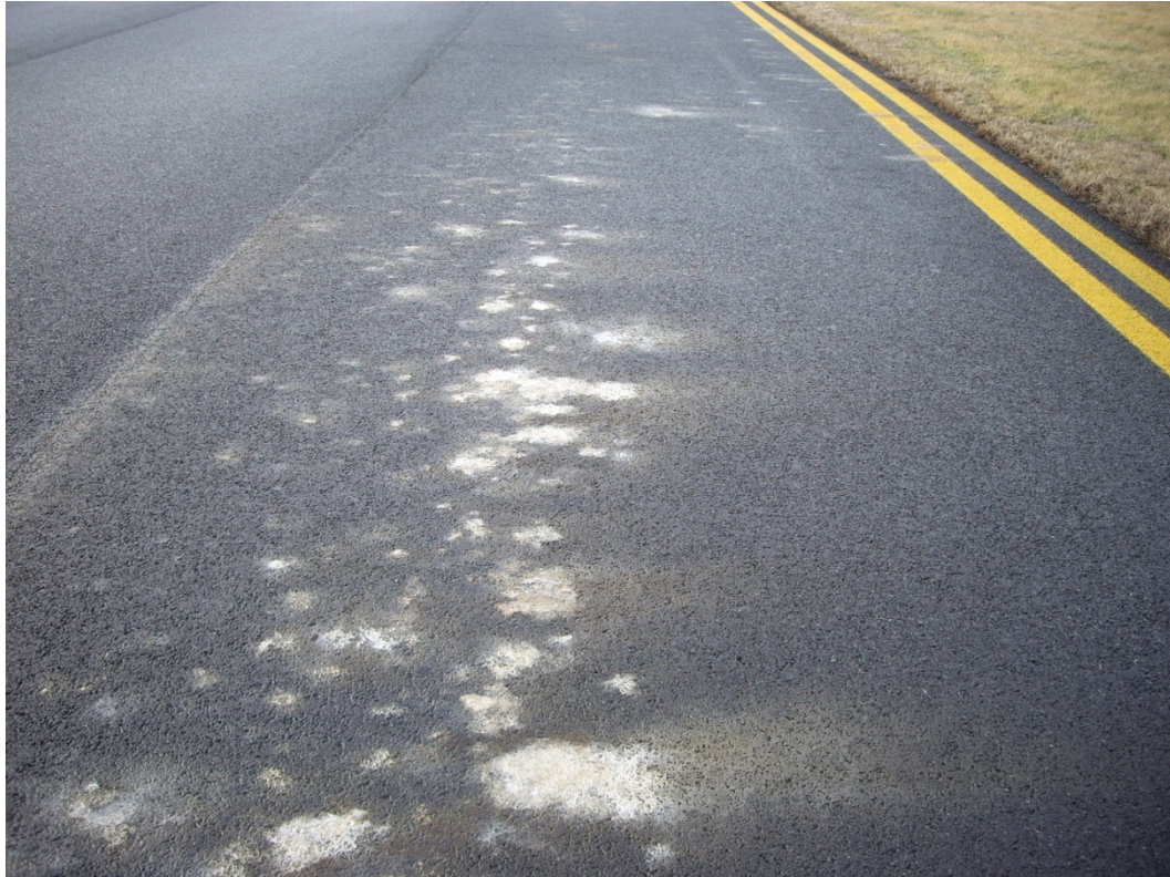
FIGURE 3.17 Stained Areas on Outside Lane.
