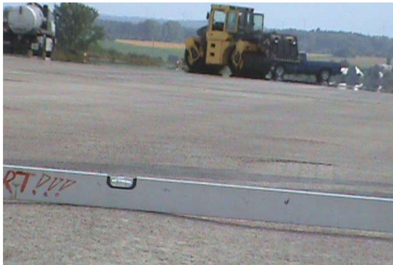
FIGURE 3.9 Small Blister under Straightedge (60).
