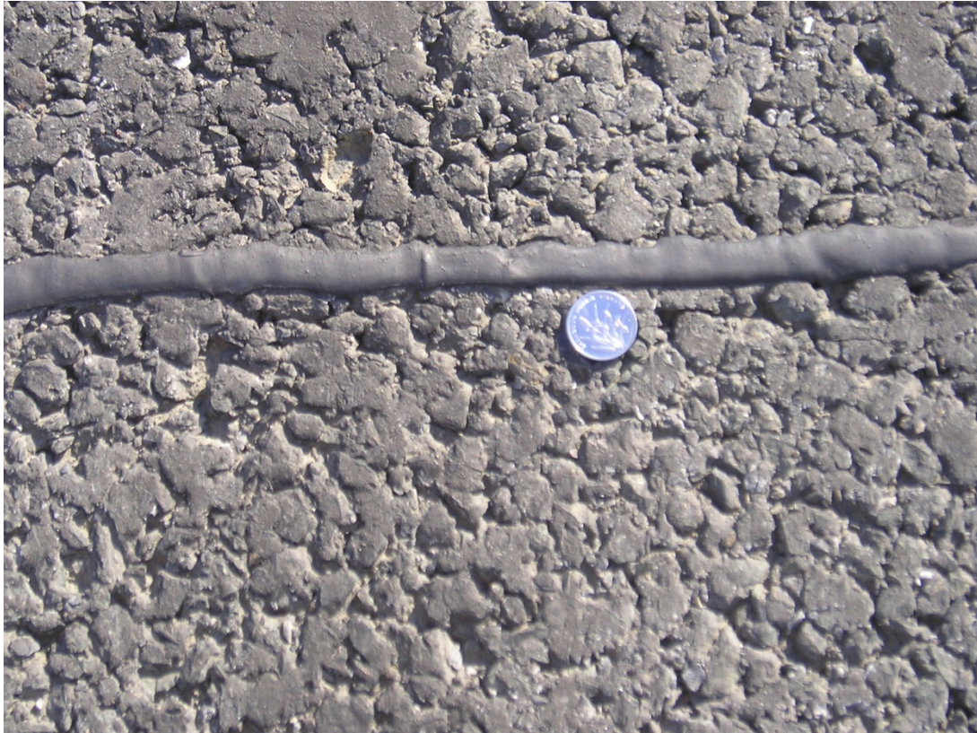
FIGURE 3.6 Apparent Thermal Crack Between Reflective Concrete Joint Crack, Harbin.
