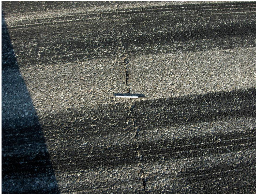
FIGURE 3.13 Transverse Crack Near the Concrete End.
