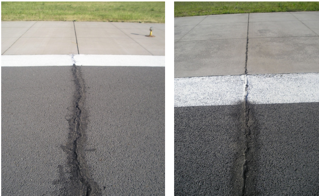
FIGURE 3.7 Transverse Reflective Cracking at Harbin.
